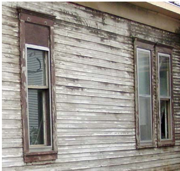
A.4.5 Inappropriate resizing, left window opening
