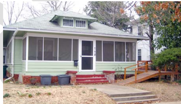
B.5.3 Example of an accessibility ramp that enters the front porch from the side. The ramp can be easily removed in the future without needing to repair the historic materials on the front elevation.
