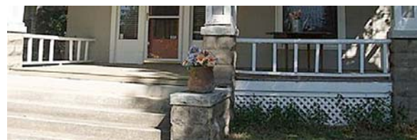
Inappropriate design – balusters too far apart.
