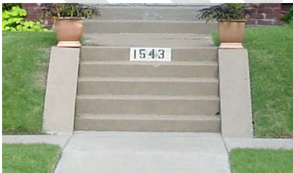
G.2.1 Bulkheads are the sloped strips of paving flanking the steps above. Note the width of the paving and how the angle is flush with the sidewalk, not raised above it.
